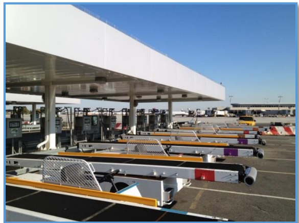
Electric Belt Loaders and Charging Stations
